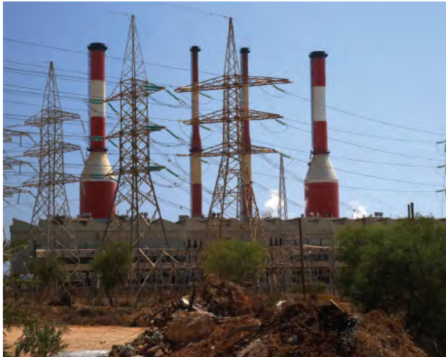
Figure 31.2: In this oil-fired power station in Cyprus, the indirect costs are a very high proportion of the total costs in electricity generation
